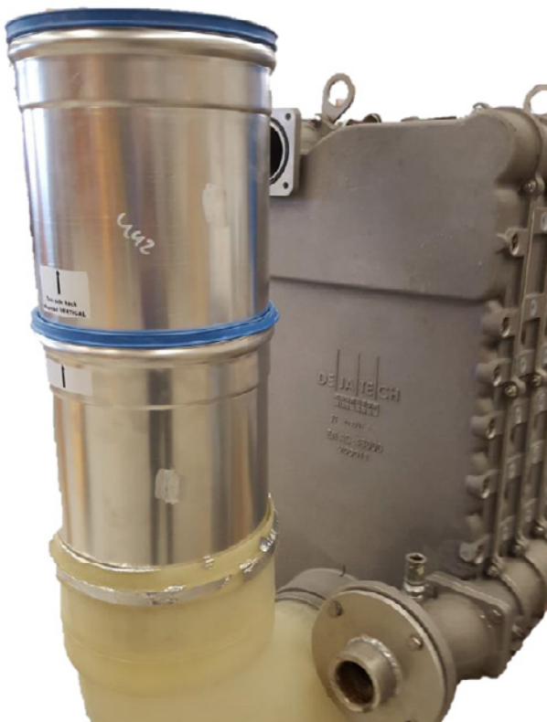
Two silencers mounted on a 5 sectional boiler (340 kW)
